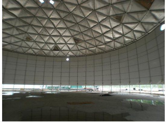
Figure 1.01a. 40 m diameter water tank was installed from grade level, using Tank Connection's jacking system.
